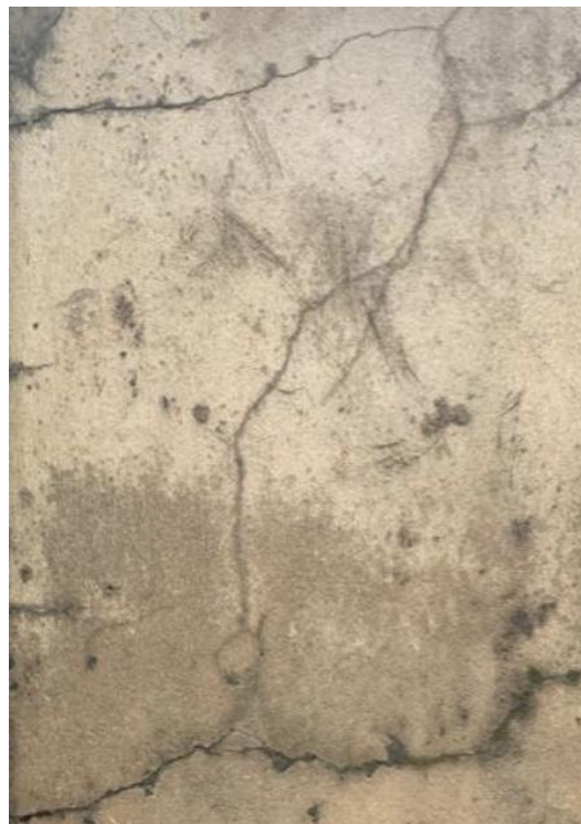
Figure 3: Plastic shrinkage crack.
