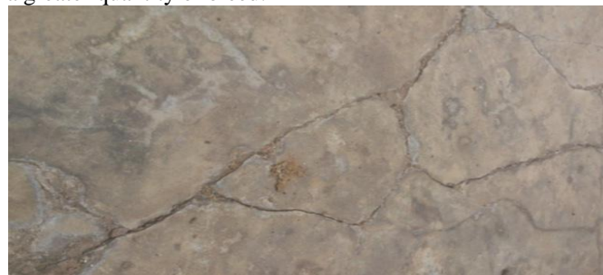
Figure 5: Drying Shrinkage crack [17].
