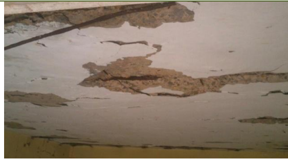
Figure 7: Steel corrosion-induced cracking
