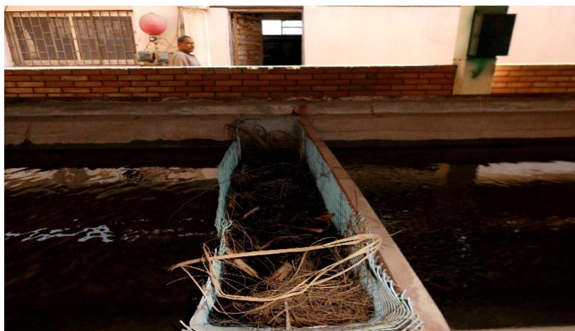
Photo 1. a The box of the accumulating weeds and debris
