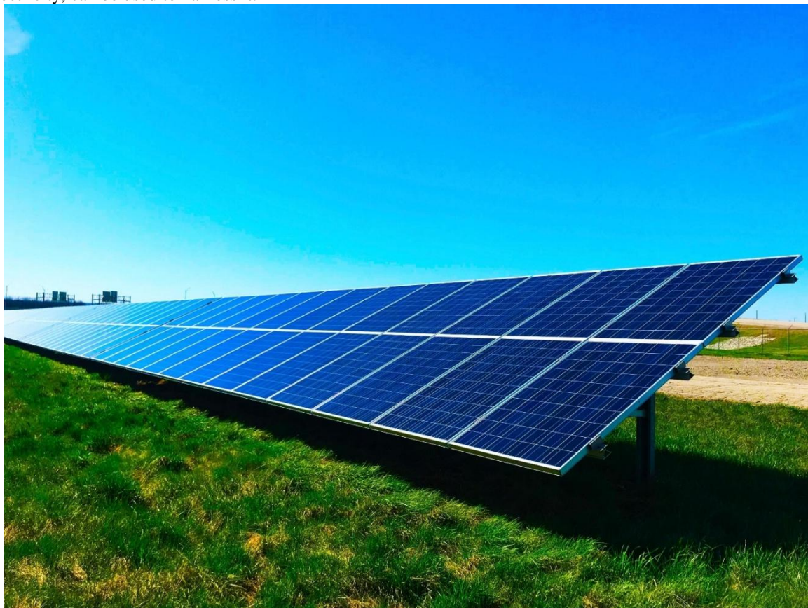
Fig 1: Solar energy panel
