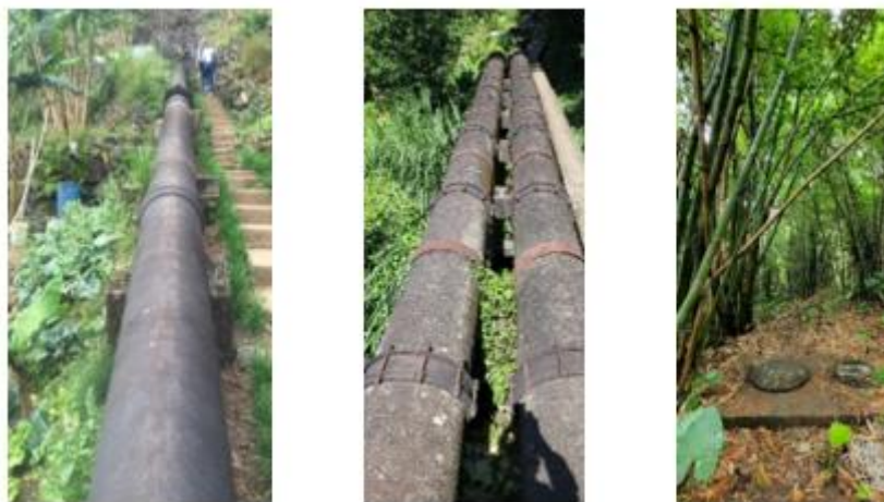
Fig. 2-1-3. Photos of \varnothing 700-mm cast iron pipe, parallel \varnothing 600-mm reinforced concrete pipes, and manholes
