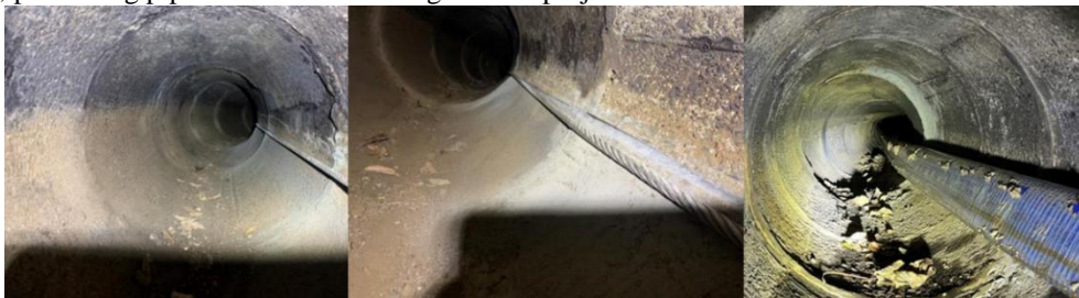
Fig. 3-1-3. Numerous bends cause slot on the RCP and scrap liner
