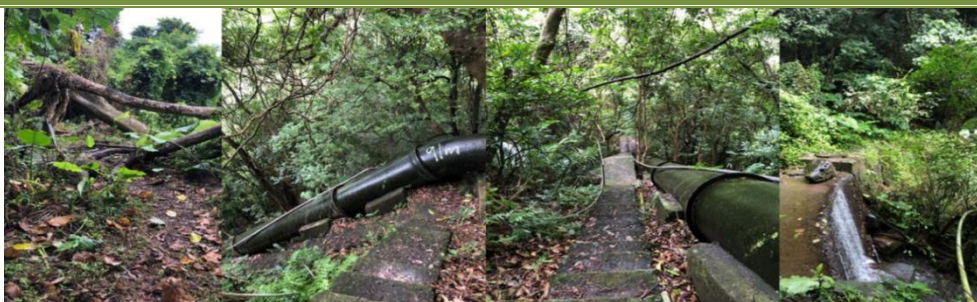
Fig. 3-2-2.4 extra 45° elbows at the siphon caused extra tensile load
