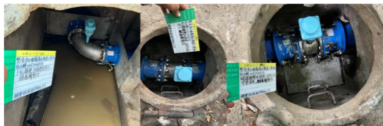
Fig. 2-4-3. Short stainless-steel tube mounted to steel plates on manhole walls.
