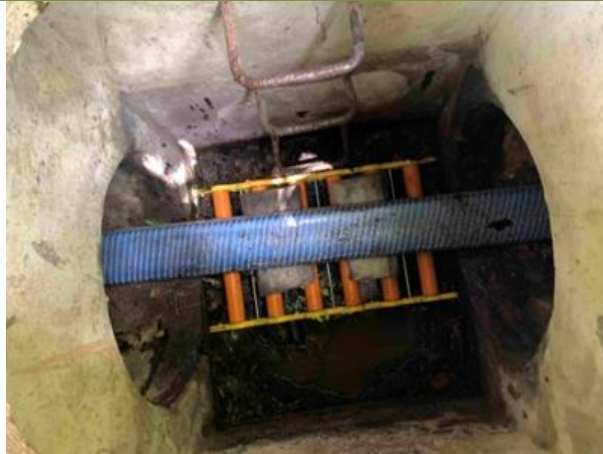
Fig. 3-3-2. Roller sets installed on the floor of manhole chambers
